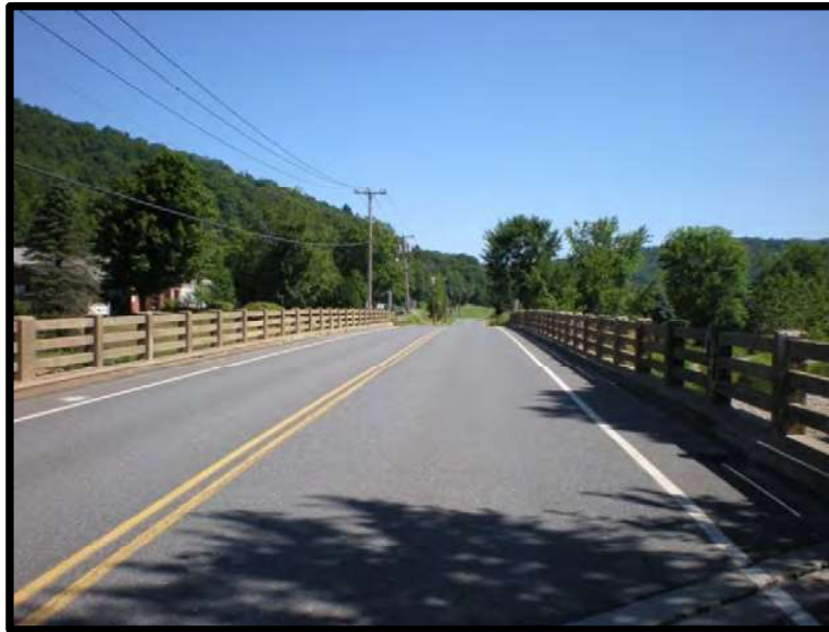
A view to the north of the bridge on Jacksonville Road (Route 112) with the Colrain Central School to the left of the bridge.
